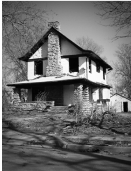
This vacant house is one of many of its kind located in what has been named "America's Most Abandoned City."
